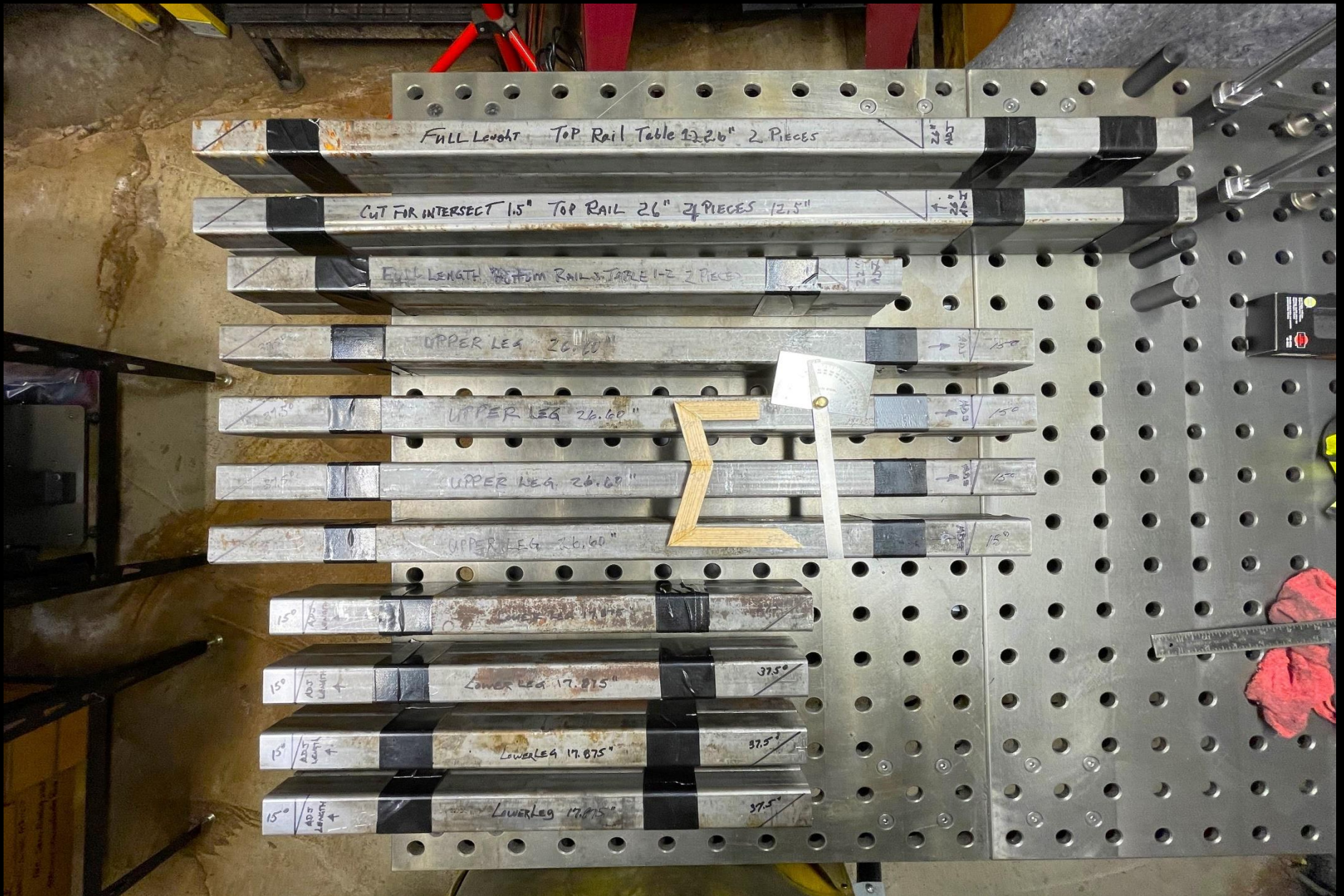
I lay out the angle and label each component prior to making the miter cuts. I will cut all of the 35.5 degree miter cuts first. I will have two drops that will be used for the splits.
