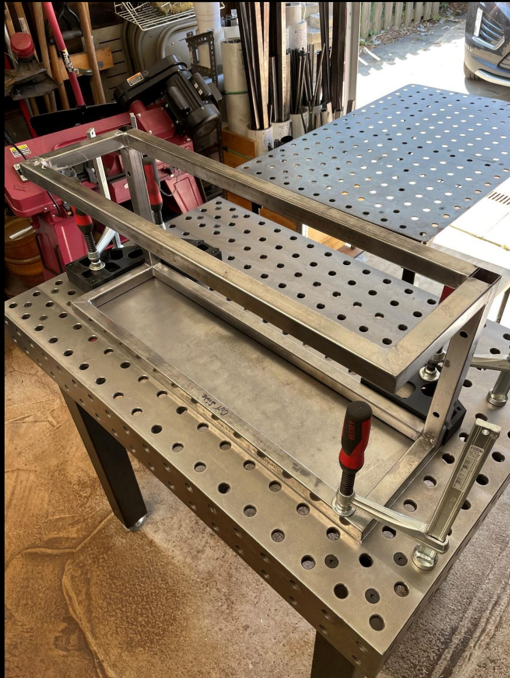
Spa Book Shelf- Fabrication Sequence: 25 Top plate is welded to the upper shelf.
