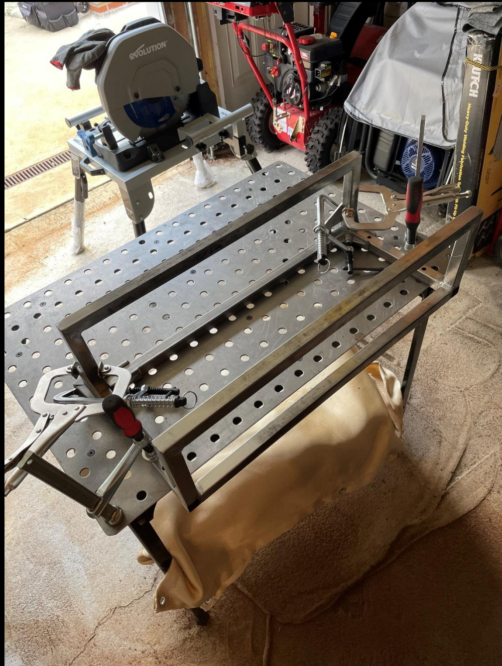
Spa Book Shelf- Fabrication Sequence: 17 Using 3 axis clamps to weld upper shelf.
