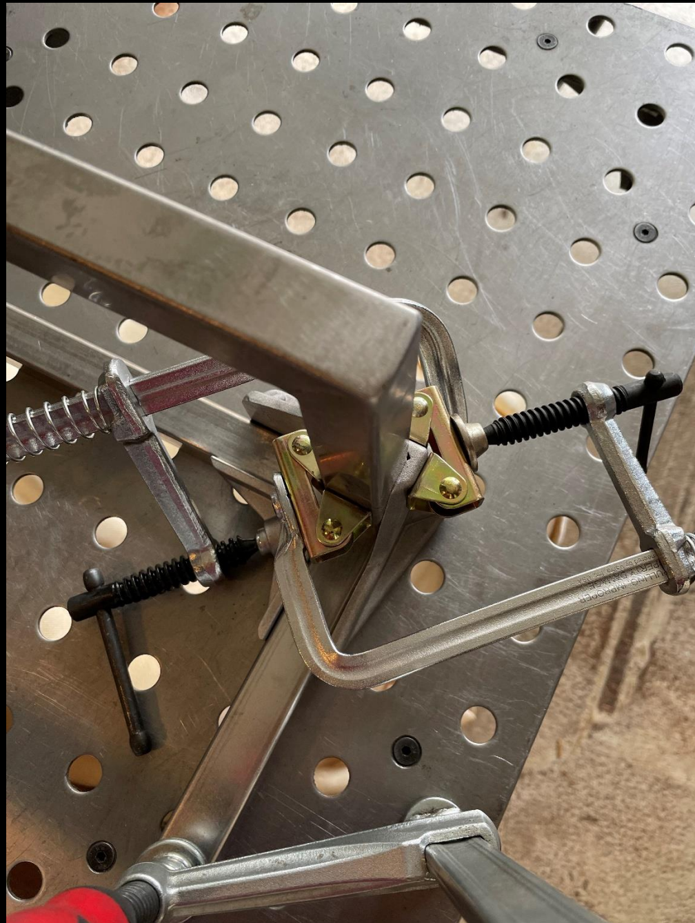
Spa Book Shelf- Fabrication Sequence: 19 Tack weld upper shelf and back-side A.
