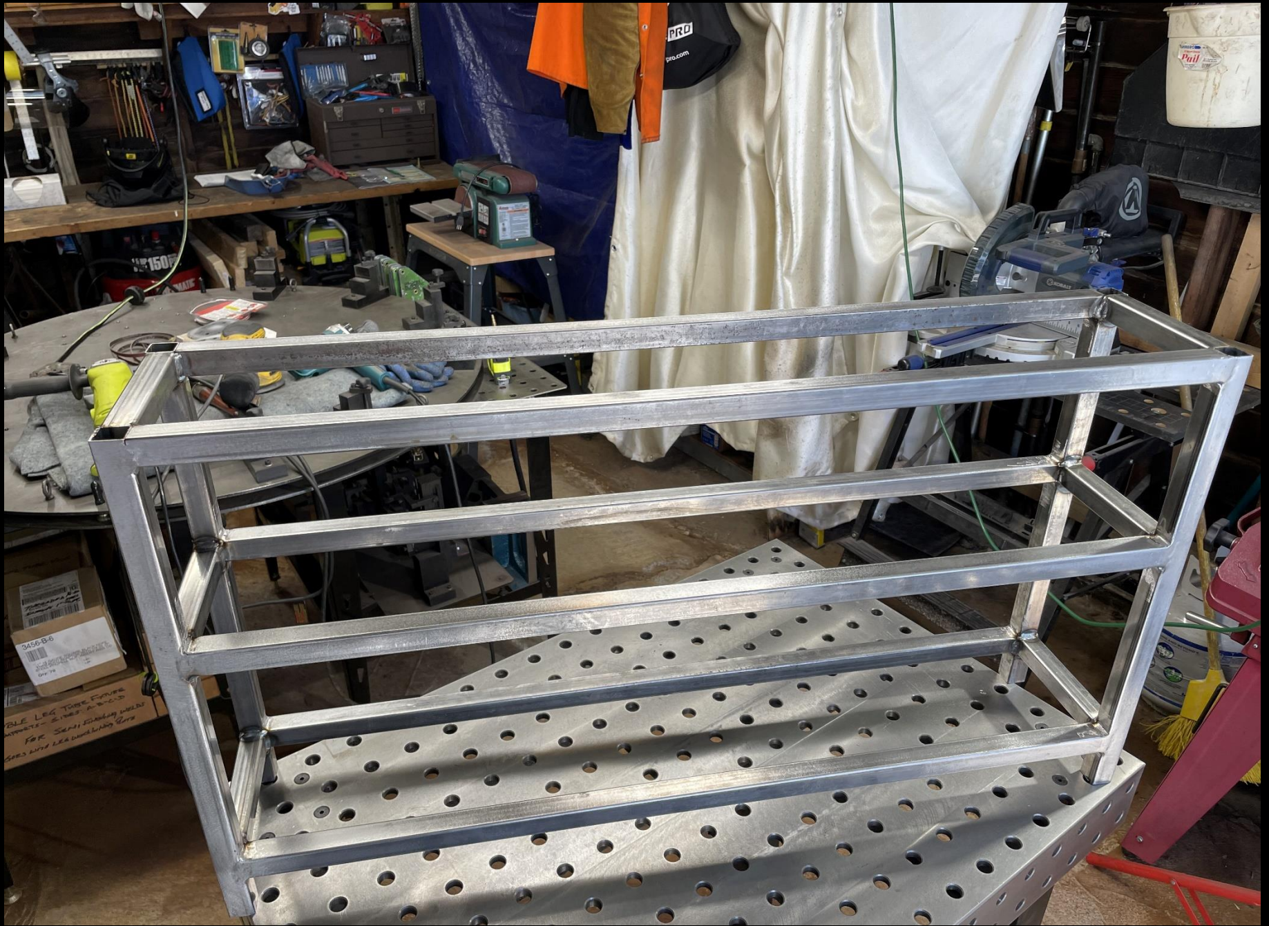
Fabrication Sequence: 16 All of the cross rail welds need to be ground and finished.
