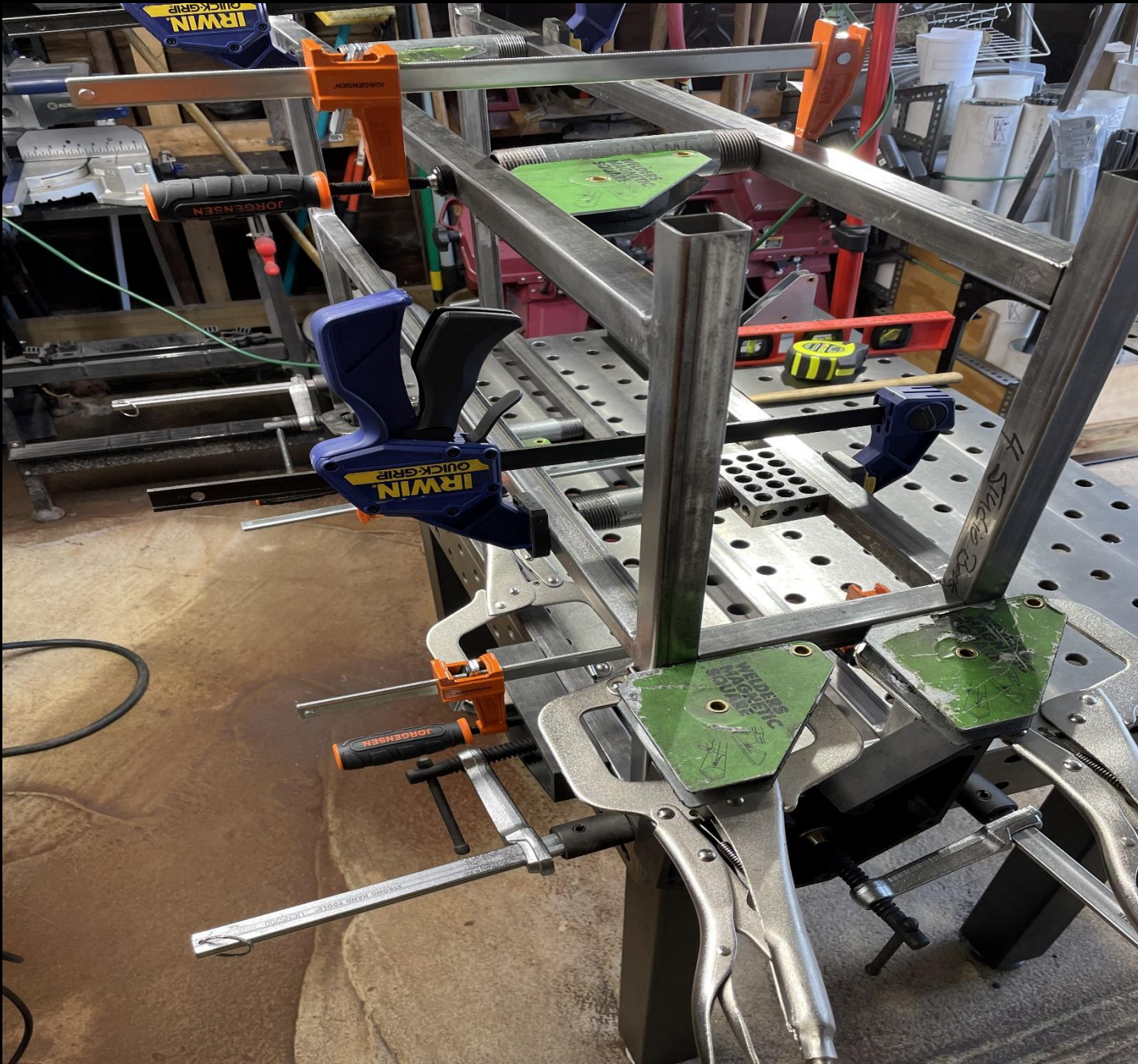
Fabrication Sequence: 11 The upper cross rails on both sides are welded first.
