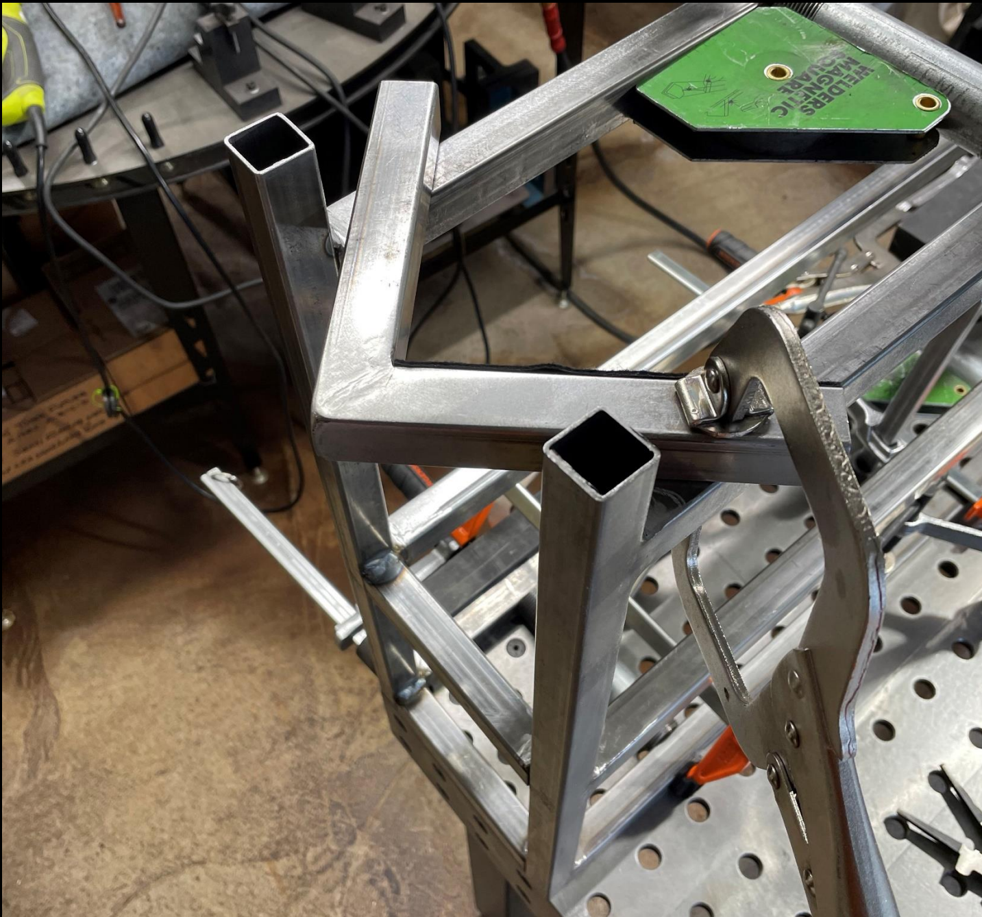
Fabrication Sequence: 14 The clamps remain in place & the lower cross rails are welded.
